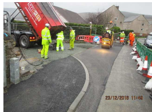
Photograph 10 – Completion of roadworks on Dixon Avenue for the new road access to the school.
