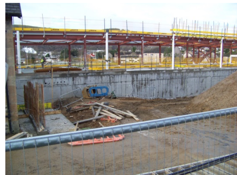
Photograph 4 Front elevation viewed from Park Road. Steel frame now linked with retaining wall
