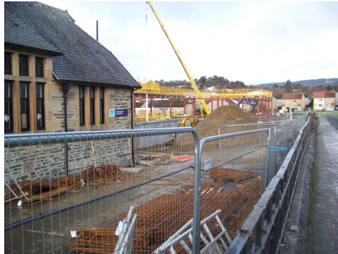
Photograph 5 Park Road elevation with retained 1881 building and sports hall frame now visible in the distance.
